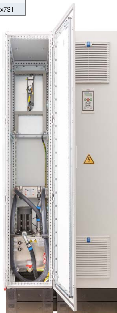
Cooling section water to water heat exchanger.
